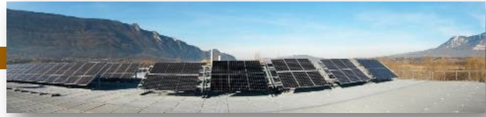
Reliability and bankability test platform
