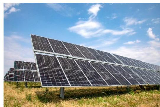
Figure 2 - Horizontal single axis tracker (1 and 2 modules) in PV utility scale plants
