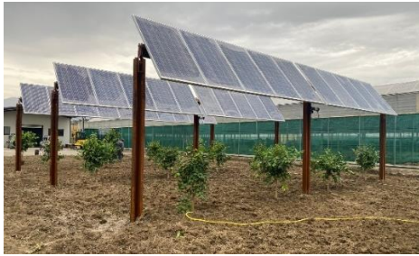
Figure 12 - AgroPV structure, Scalea
